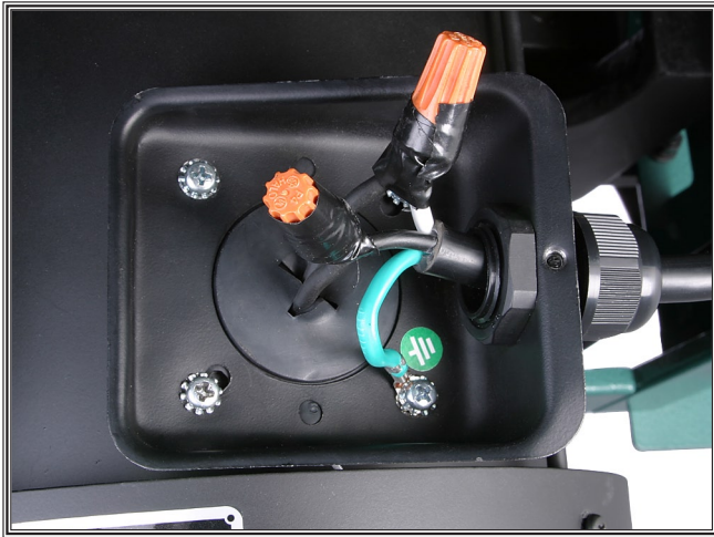
Figure 78. W1761 motor junction box, 220V single-phase.
